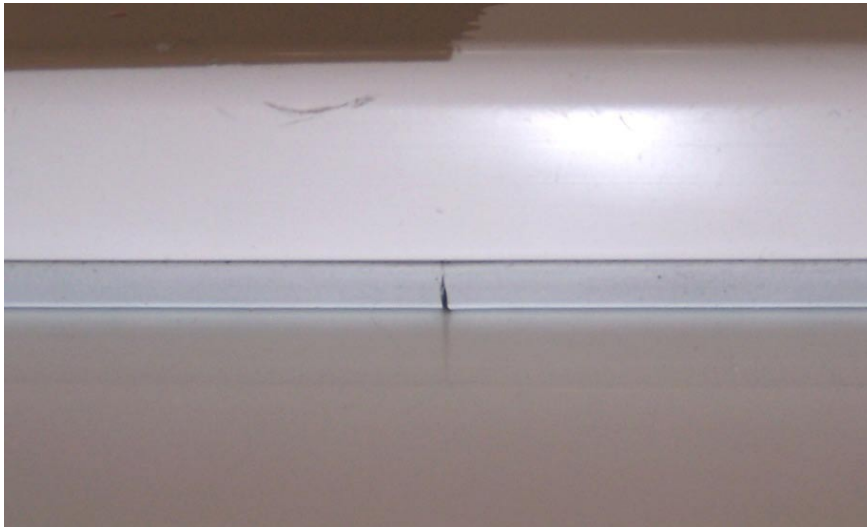
Figure 16: Leakage in the longitudinal join of one EPDM gasket upon conclusion of the test cycle
