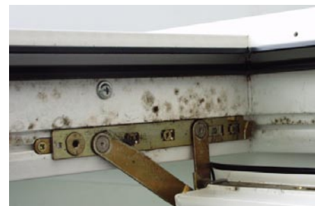
Figure 3: Mould growth in the upper frame rebate (PVC window)
